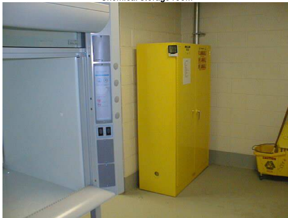
Chemical storage room
