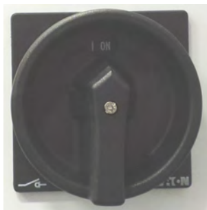
Power Switch On
