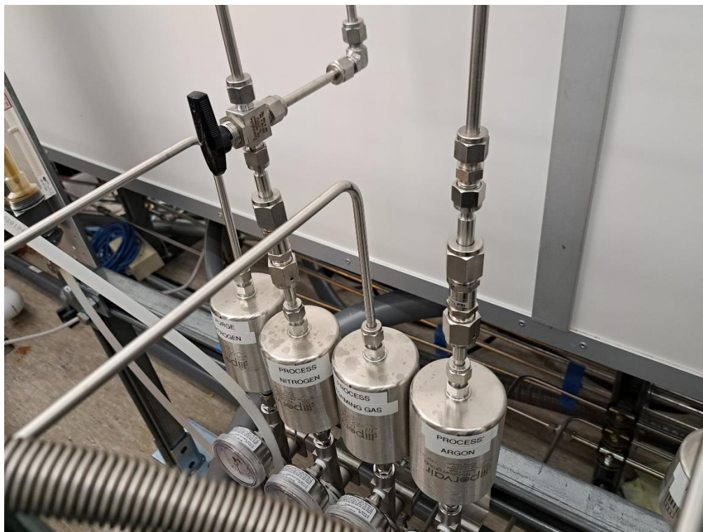
Figure 1: Gas valve set for processing with N 2
