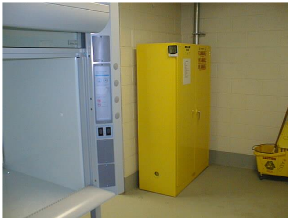
Chemical storage room
